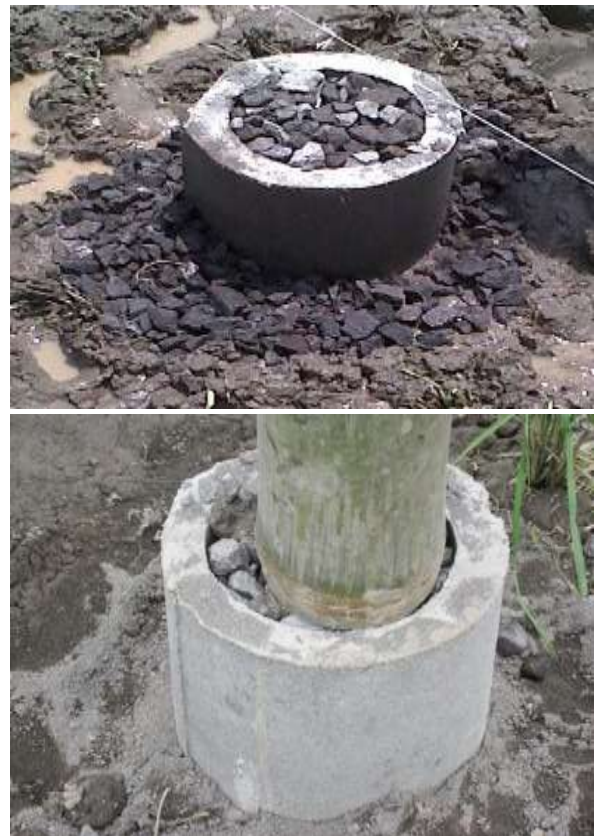
Fig. 3. Hollow Pedestal Foundation Before and After the Bamboo Column was Put on top
