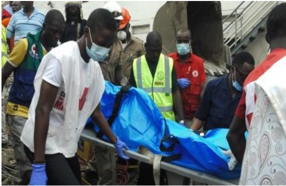
Figure 7. Four persons, including a 15-year-old hawker identified only as Sukurah, lost their lives after a two-storey building under construction, collapsed in Surulere, Lagos State. (Source: http://urbanpostng.com/news/photos-4-killed-in-lagos-building-collapse/ )
