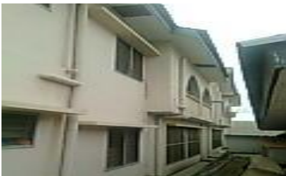
Plate 4. A Students' Hostel with inadequate side setback and open space wide enough for only concrete rain water drainage.
