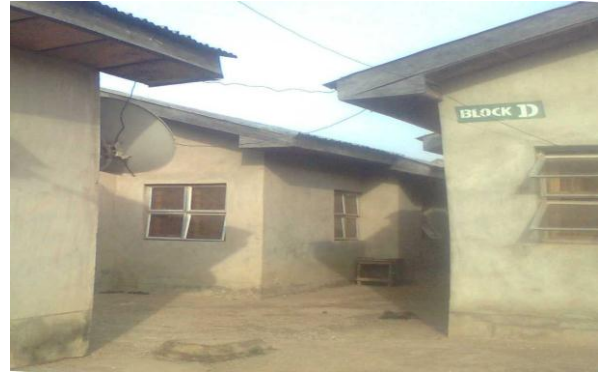
Plate 5. A Students' Hostel with inadequate setback between blocks and concrete paved open spaces without any soft landscape element.
