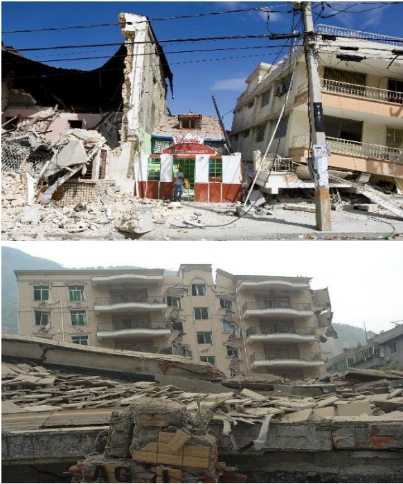
Fig. 4. Building damage to column failure (left) and beam failure (right) (photo: Marco Domino)
