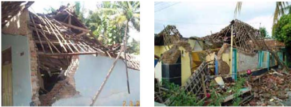
Fig. 11. The broken brick walls (photo: Boen)
