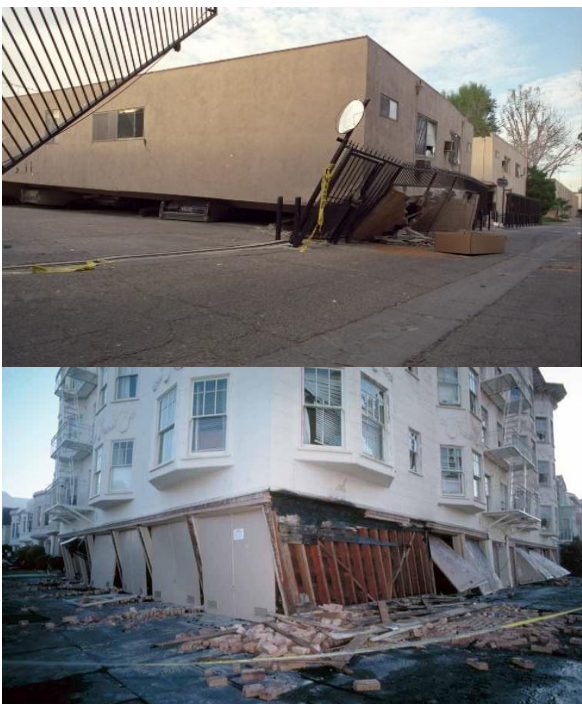
Fig. 5. The impact of the earthquake due to the soft story effect on the building ground floor (photo: Gedstrom and Nakata USGS)
