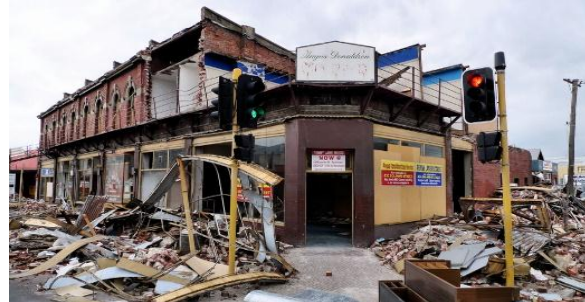
Fig. 8. The asymmetric plan makes the torsional effect on the building (photo: Martin Luff)
