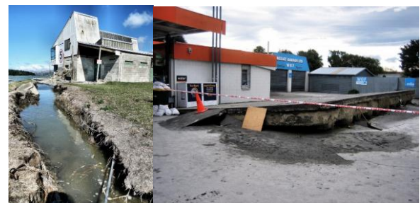
Fig. 10. The foundation failures due to the ground (left) and the liquefaction effect (right) (photo: Martin Luff)
