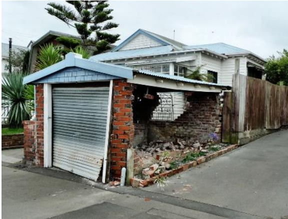
Fig. 2. Low buildings damaged resonated with the high frequencies (photo: Martin Luff)
