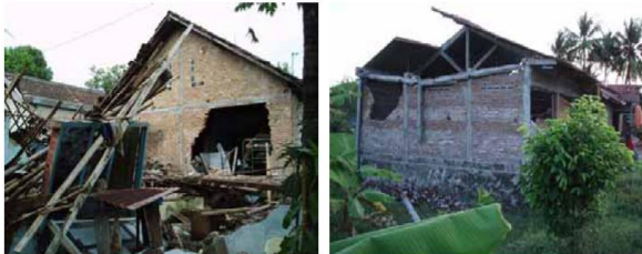
Fig. 12. The broken concrete frames (photo: Boen)
