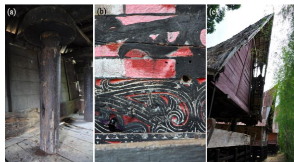
Fig. 6. (a) Holed pole in Sopo (b) A beetle tries to hole Gorga (c) Decayed fibers roof at the oldest Sopo (S4)
