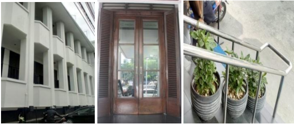
Fig. 15. Balcony on right side of building, glass material at door, and steel material in railing
