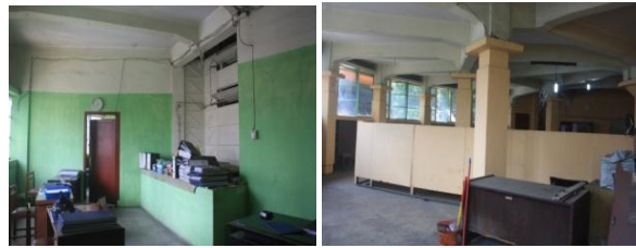
Fig. 9. Room Atmosphere that shows natural light into the PD Pasar office Medan
